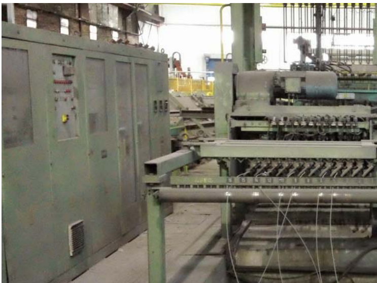
Control Cabinet with Function Control and Weld Processor
